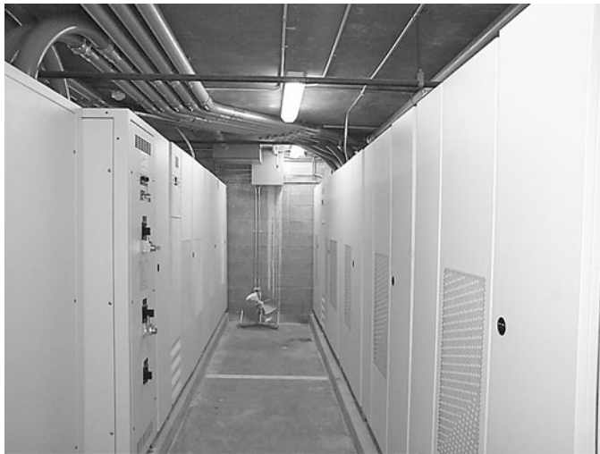
Figure 6.1 A modular UPS at GNAC, Inc.
