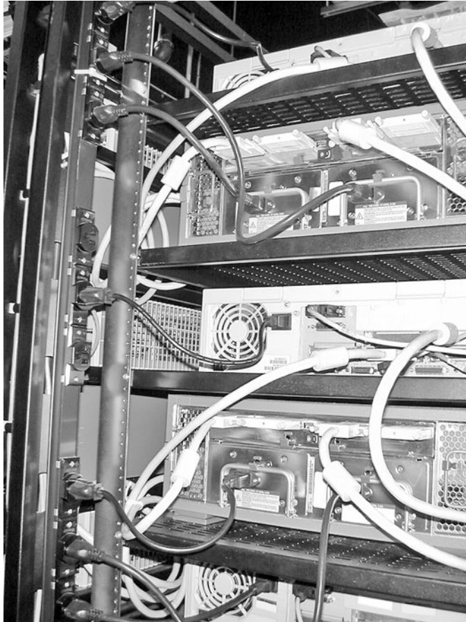
Figure 6.18 GNAC, Inc., brings three legs of UPS power into a single power strip. Redundant power supplies in a single piece of equipment are plugged into different legs to avoid simultaneous loss of power to both power supplies if one leg fails.
