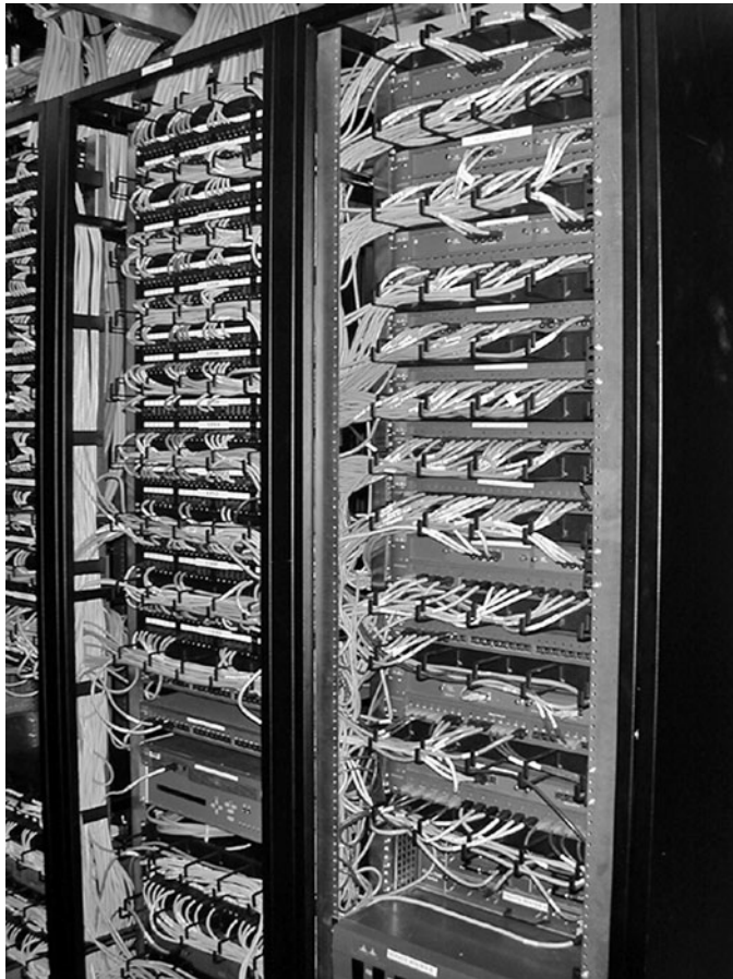
Figure 6.11 Network racks at GNAC, Inc. (Patch panels are connected to overhead cabling to prewired patch panels at the top of each host rack.)
