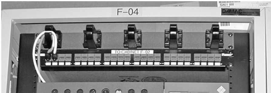
Figure 6.9 Racks at Synopsys are clearly labeled at the top and have a patch panel that indicates the rack to which it is wired.
