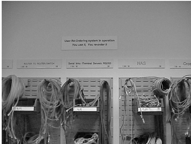
Figure 6.17 Eircom uses a mixture of blue bins and hanging cables.
