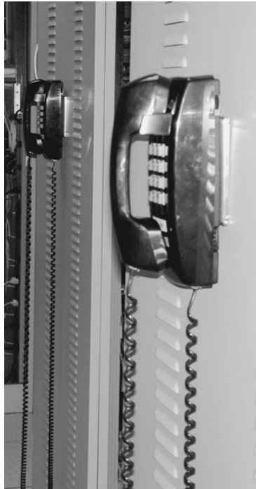
Figure 6.14 SAs at Synopsys all have radios but find that phone extensions at the end of each row work better in the data center. (Note the extremely long cord.)
